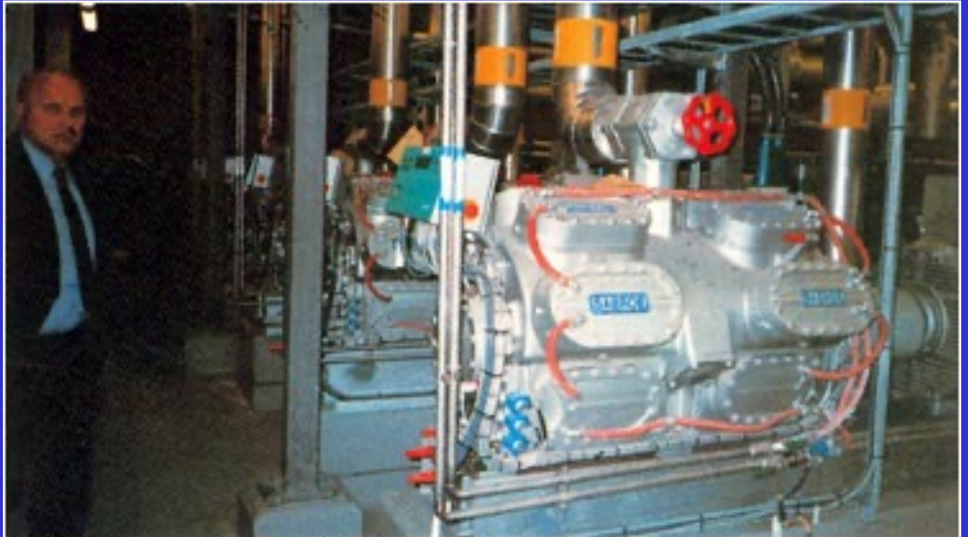
HVAC Plant Room at Oslo Airpoprt, Norway
