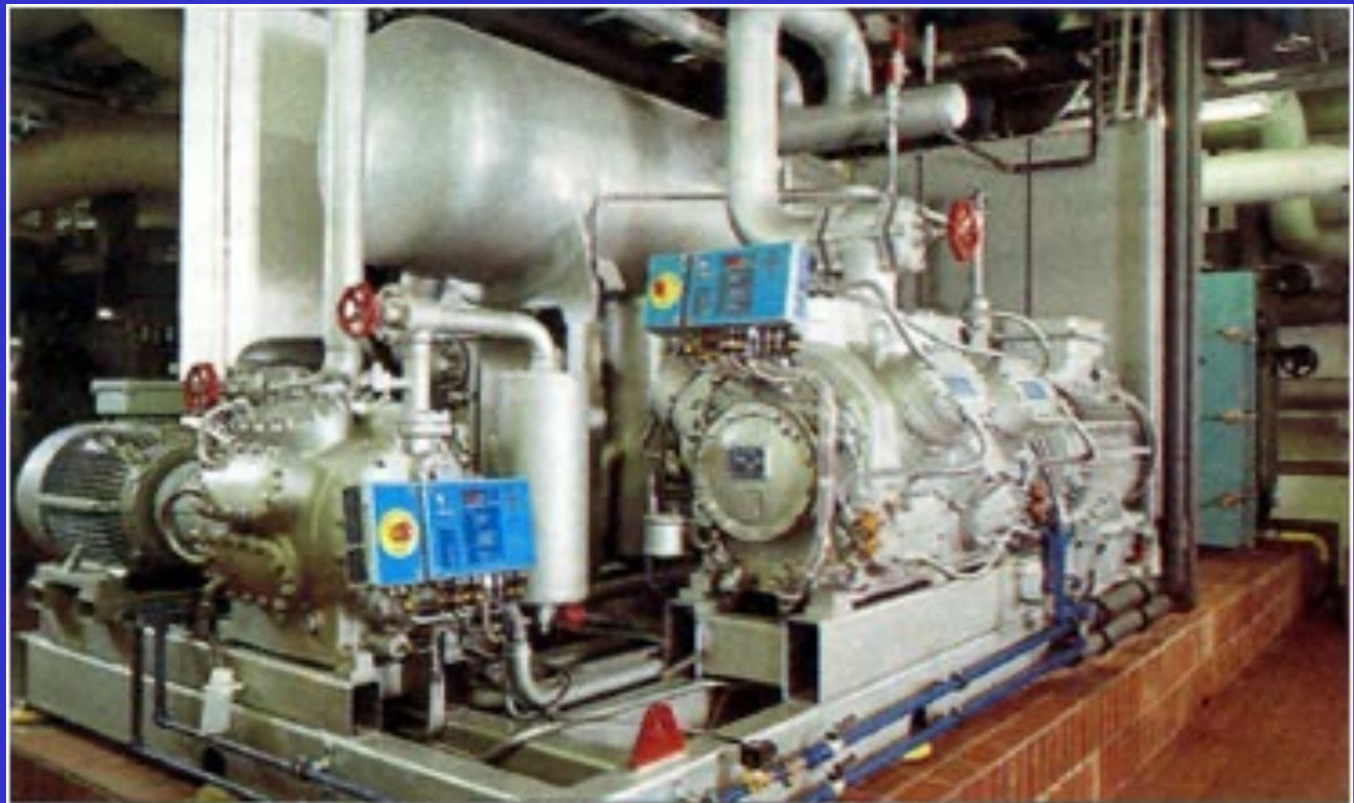
The complete Ammonia Chiller package including electric starter panel and all wiring at the P&T building, Copenhagen.
